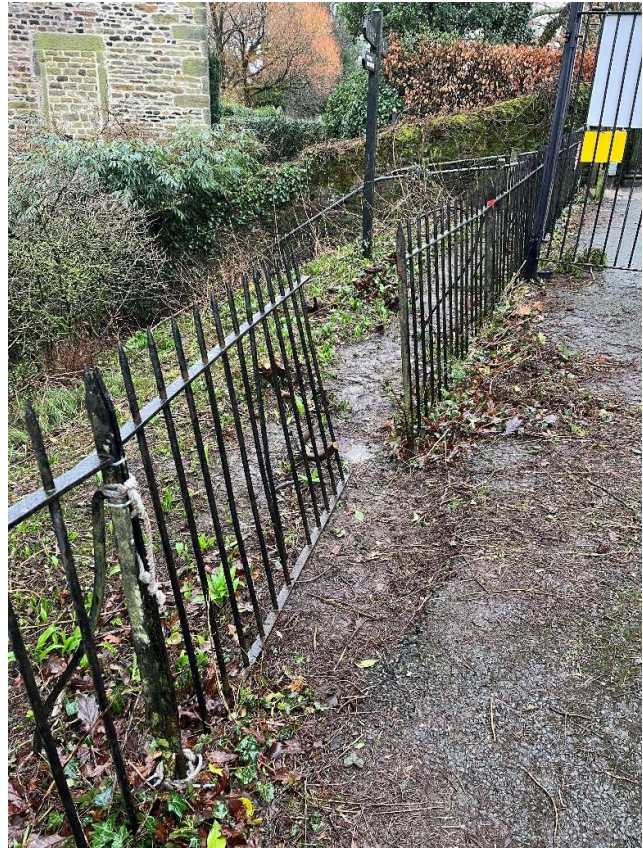
Photo 4. – This section of railing is now missing...!
