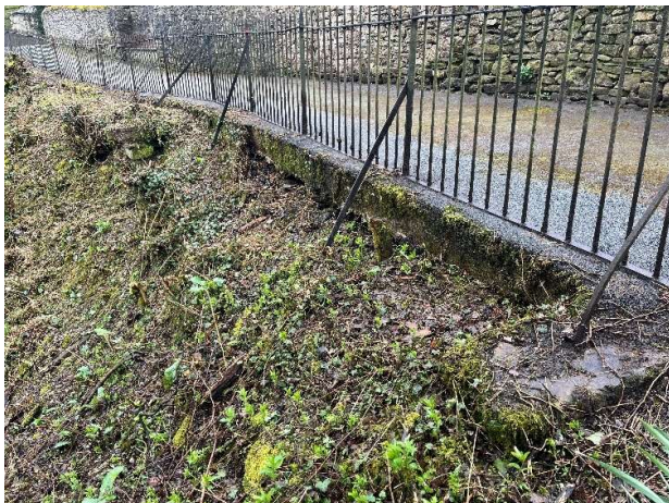
Photo 1. – Undercutting of footpath.
