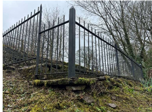
Photo 2. – No support under corner of North platform.
